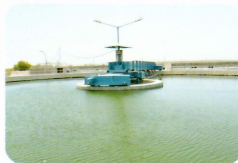
Clarifier Bridge Section at Water Filtration Plant, Jacobabad
